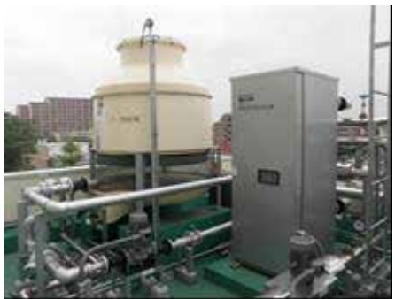
温水焚吸収式冷温水機(右)
