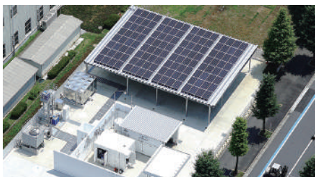
Example of utilizing Green Hydrogen (refueling equipment for fuel cell forklifts)
