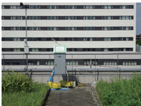
View of monitoring equipment
