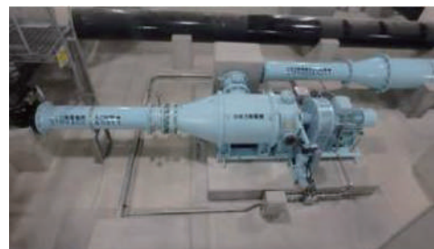
Small hydropower generation equipment
