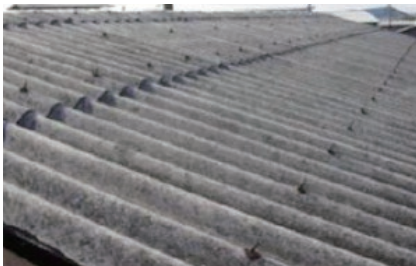
Asbestos-containing slate (wave slate)
