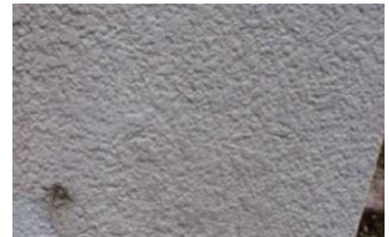
Asbestos-containing texture coating (stucco exterior wall)
