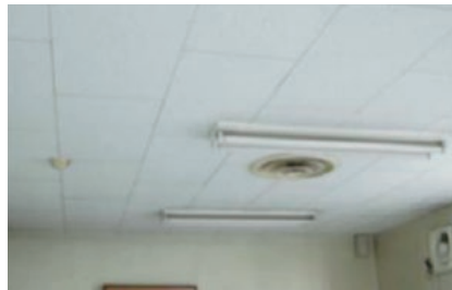
Asbestos-containing ceiling tiles (ceiling)
