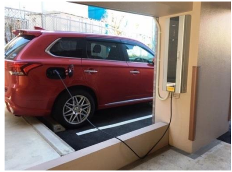
Example of EV charger installed at multi-family housing
