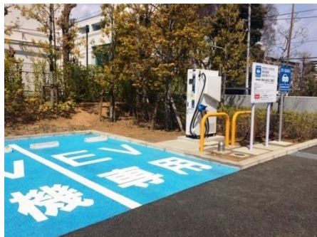
Public EV charger at TMG-owned facility (Tachikawa Joint Government Building)
