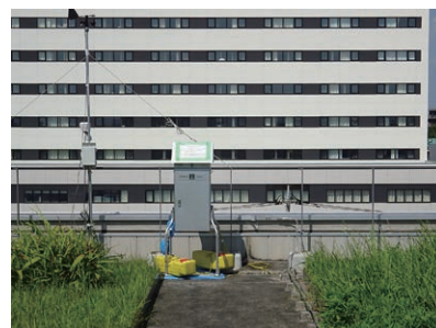
View of air monitoring
